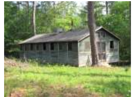
Barracks Building of the CCC Camp at Hard Labor Creek State Park in need of preservation.
